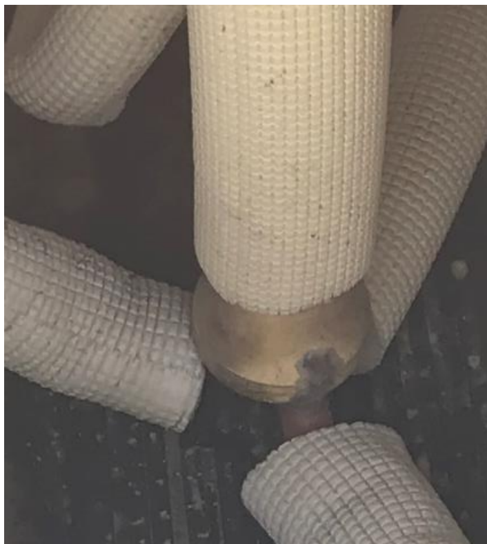
Figure 3.31 Picture of distributor
