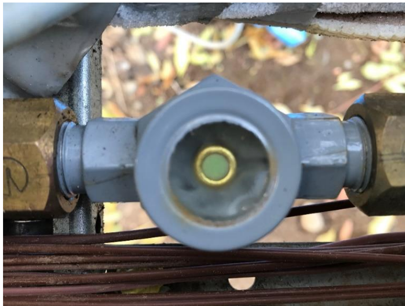
Figure 3.18 Picture of sight glass
