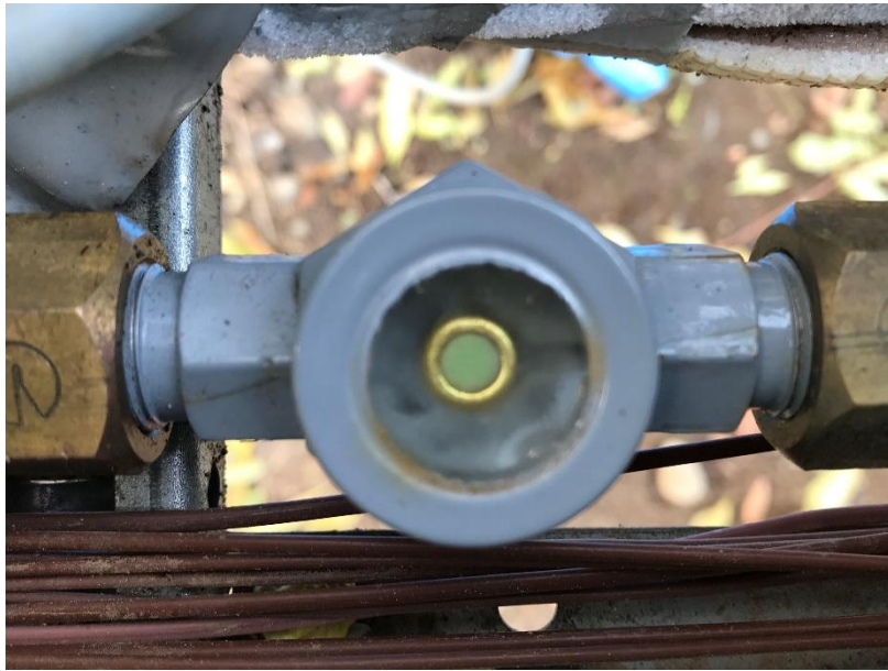
Figure 2.6 Picture of sight glass
