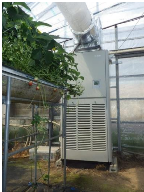
Figure 3.41 Picture of indoor unit and duct
